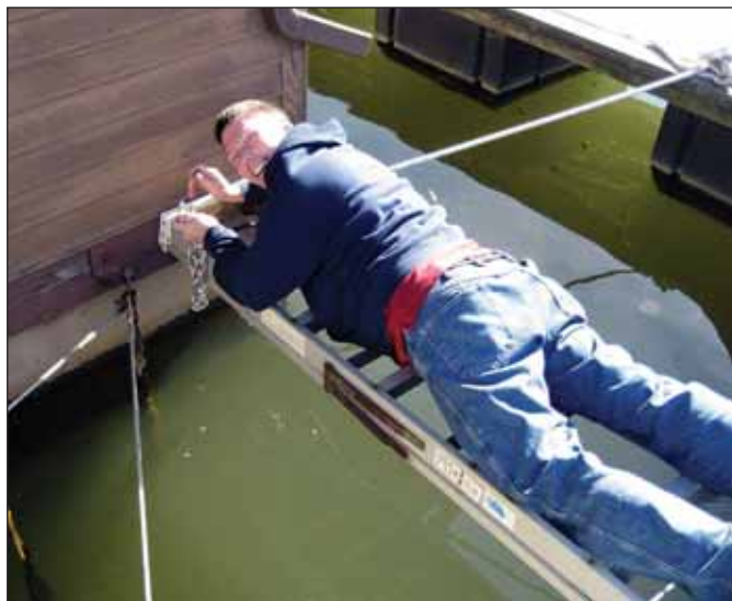
Right tool for the right job? CWO Roger Steinkemp lays across a ladder to install chains from the Association Office to the pier.
